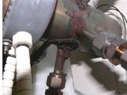
FIGURE 10. Example of corrosion damage in a LiF-NaF-KF eutectic (FLiNaK) loop component.
